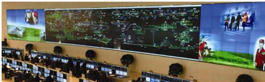
Seamless Video Wall Control Room Systems
